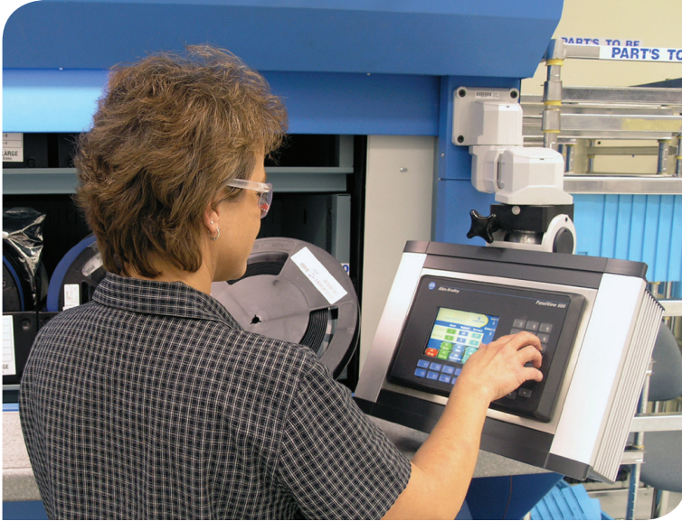
MicroLogix 1500 controllers including a Panel View operator interface allow the vertical carousel to present the correct reel with a push of a button.
